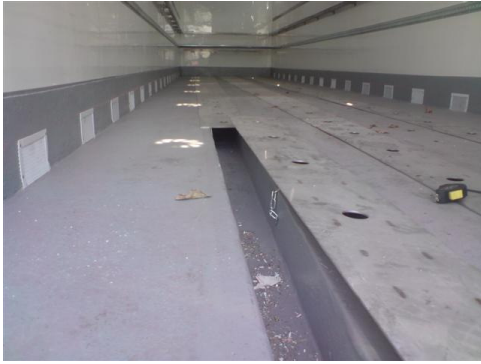
Ducting, steel cover removed. Emergency vents on each side.
