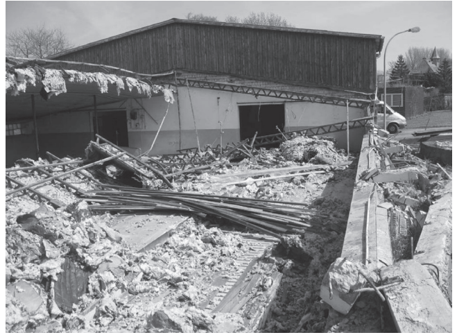
Figure 2.4.2.1.1: demolition of a cattle building: Mixture of old building materials has to be sorted due to contemporary environmental regulations.
